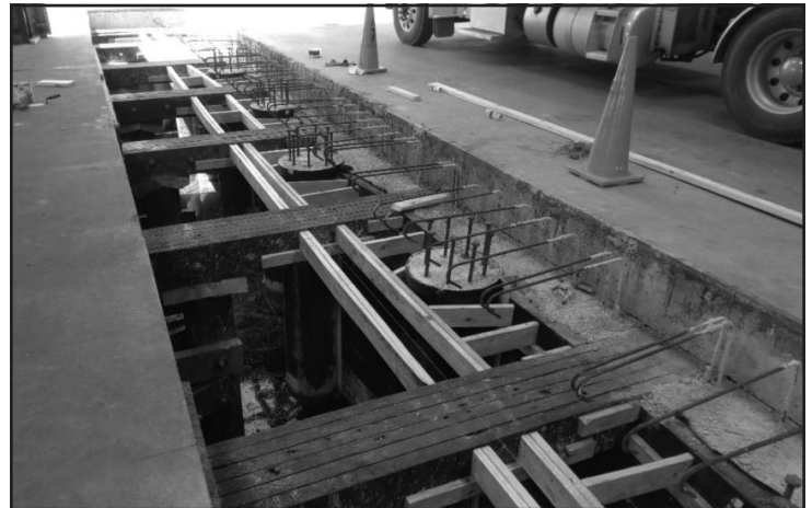
Figure 8. Beginning stages of concrete beam rebar layout after pouring the new concrete wall
