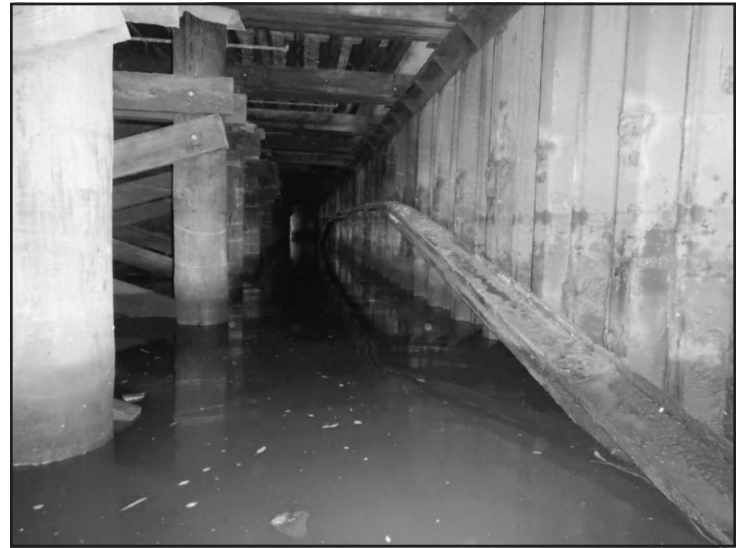
Figure 4. Existing steel bulkhead wall at Berth 9. Note failed tie rod/waler and connection of timber pile caps to top of wall
