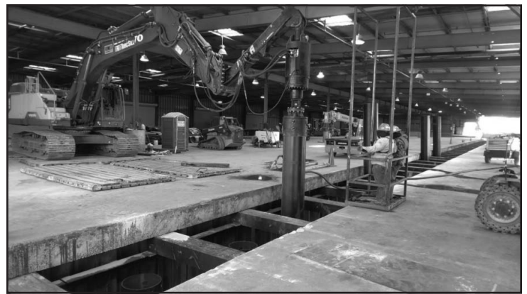
Figure 5. Helical pile installation. Note torque head fitted to excavator, piles installed between intact timber pile caps, and low clearance
